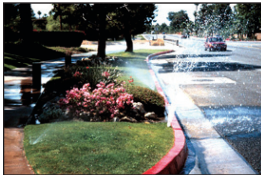
Figure 1 - Broken sprinkler floods street.
