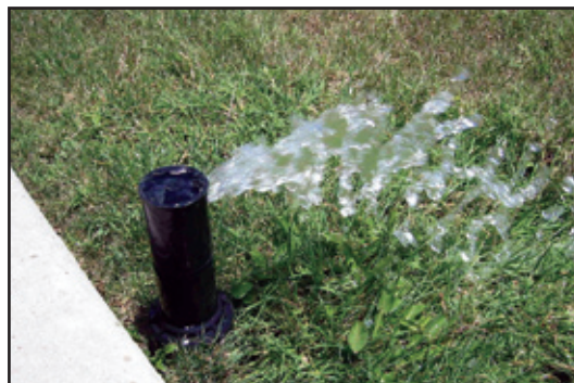
Figure 6 - Sprinkler hit by lawnmower.
