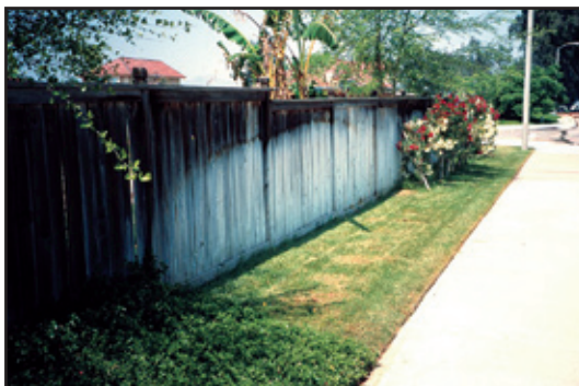
Figure 5 - Wood fence bleached by sprinkler spray.
