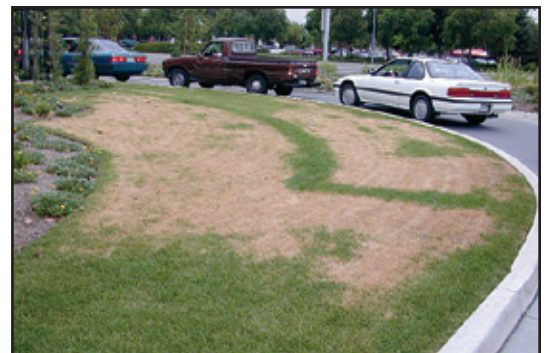
Figure 4 - Misplaced sprinklers and trenches not properly compacted.
