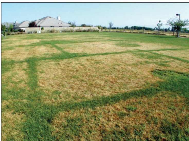
Figure 33 - Example of a sprinkler system where the trenches were not properly compacted after the PVC pipe was installed.
